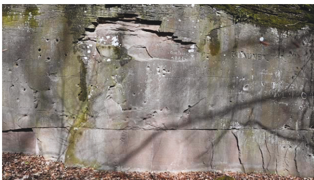
Figure 4. Stone wall with graffiti, bullet holes and a big spalled part.
