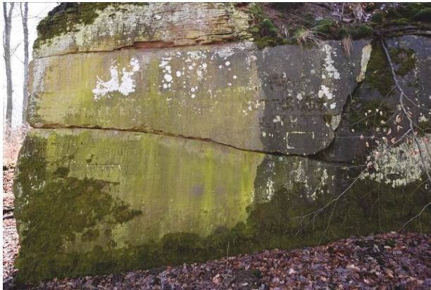
Figure 3. A stone wall of the quarry with graffiti and biological coating (moss, lichen, small tree) and water drainage traces especially on the right side.
