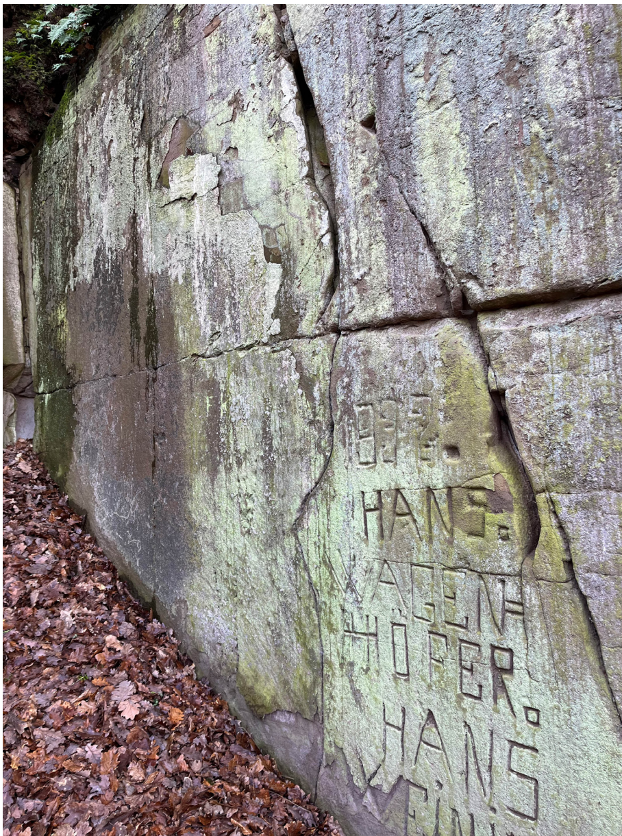
Figure 7. Area of the stone walls of the Fingalshöhle showcasing deterioration caused by weathering and the overgrowth with lichens, algae and moss.
