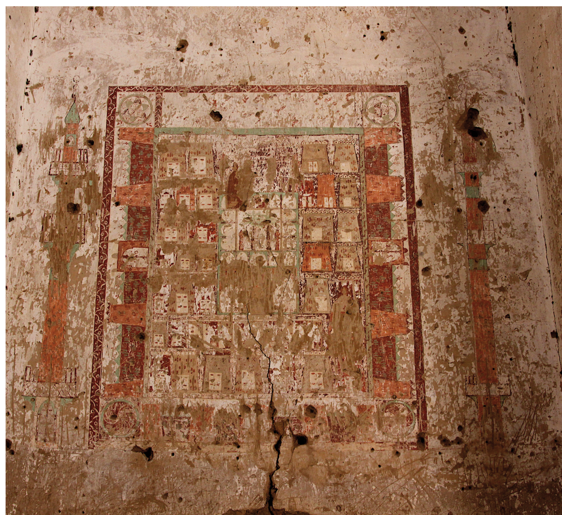
2 Vandalised and deteriorated wall paintings featuring a sacred landscape at the Gunbad mosque of Azadan near Isfahan. (Photographer: Ana Marija Grbanovic)
