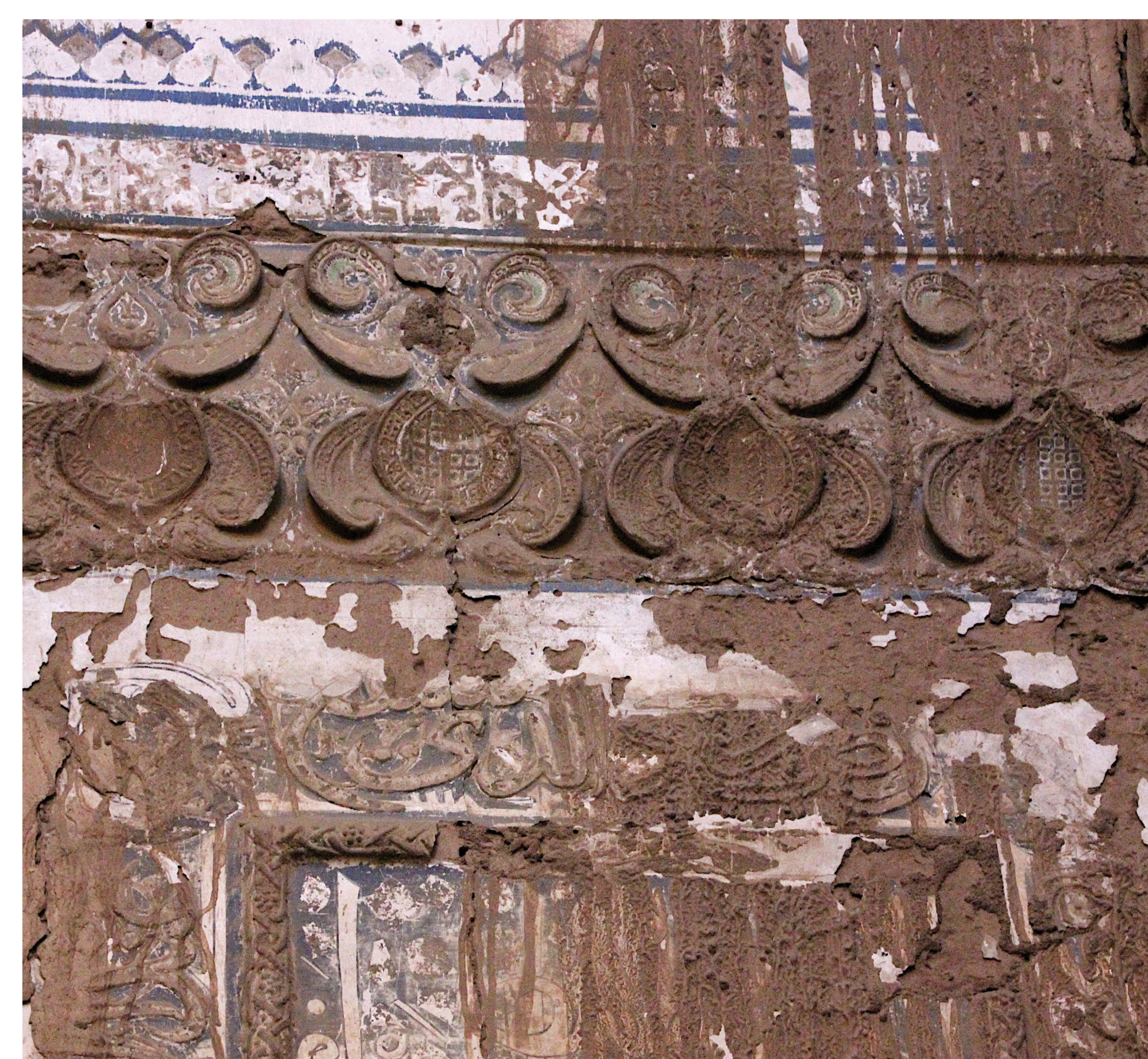
3 Badly damaged architectural revetments of the Shamsiyya madrasa in Yazd, central Iran. (Photographer: Ana Marija Grbanovic)
