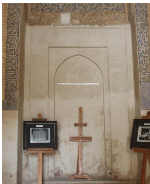
Image 11. current condition of mihhrāb 2014
