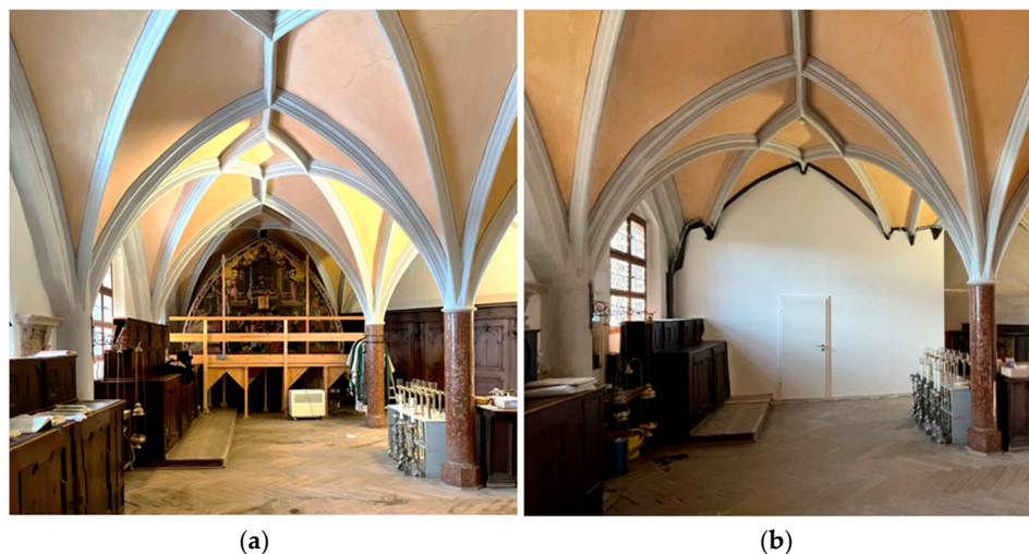
Figure 6. Working platform with panel painting in the sacristy (a,b) enclosure of the panel after the building in drywall construction (Volume: \sim 126 \text{ m}^3 ) [© BLfD, Theresa Hilger].
