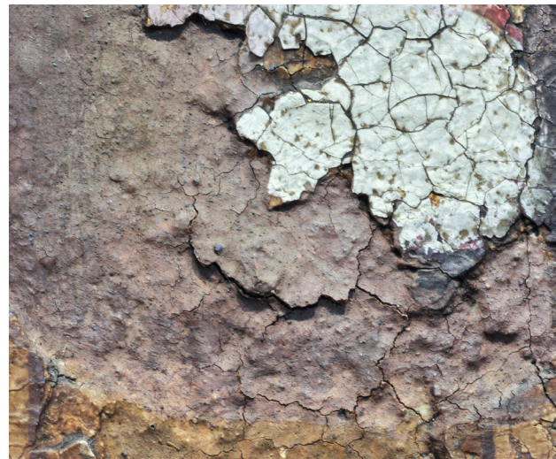
Fig. 2: Detailed view of a monitoring area with a protruding paint patch [Hoepner 2015].
