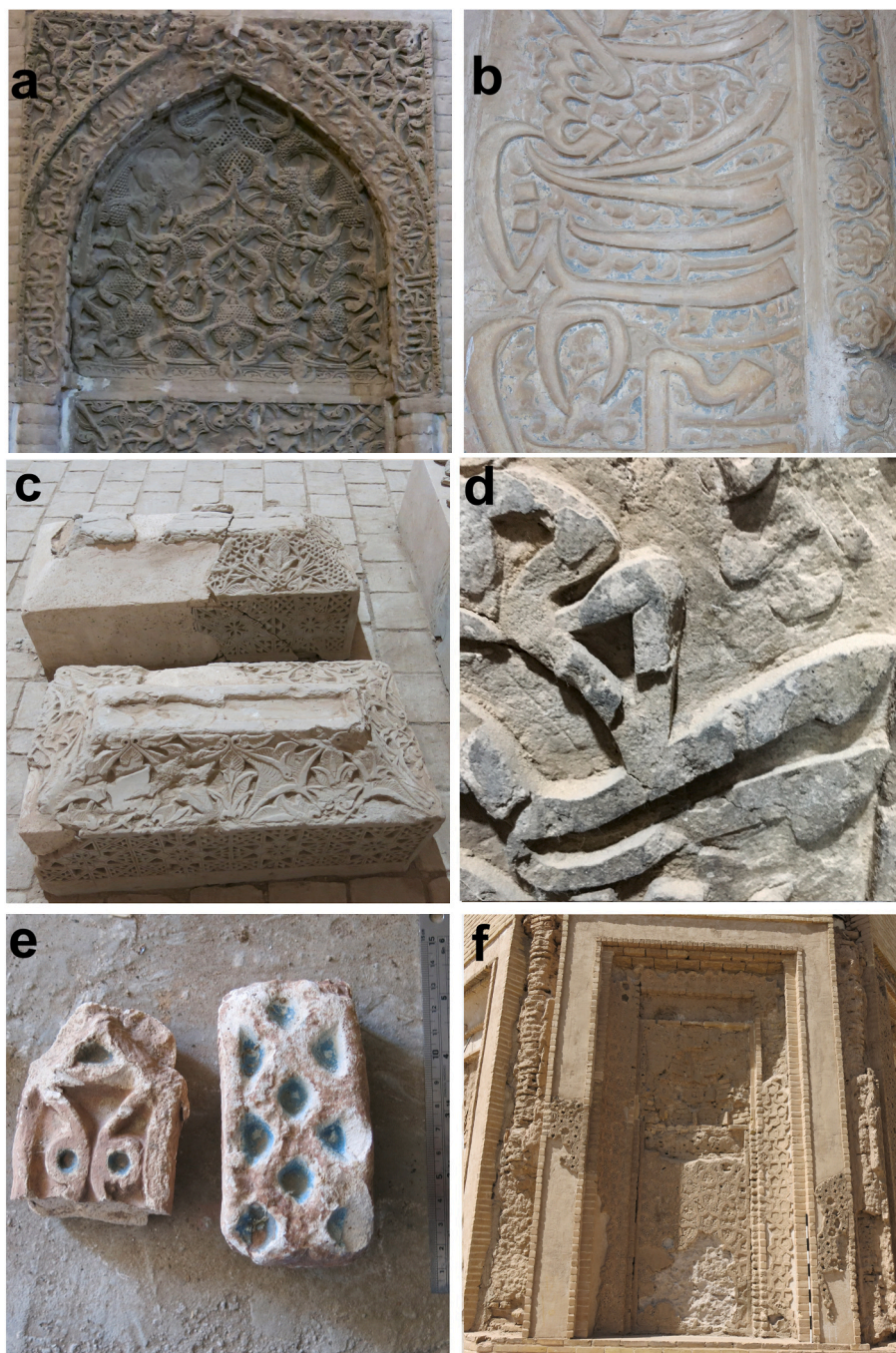
Fig. 8. Six samples of stucco decoration subjected to the multi-analytical study, a) the small mihrab in the Great Mosque of Ardestan/Loc.28, b) the stucco inscription with applique plaster technique ( fetilehiy ) in the mihrab of Jame mosque of Oshtorjan/Loc.37, c) the narrow space between stucco-decorated graves in Baba Abdullah mosque in Nayin/Loc.31, d) two distinct layers of gypsum plaster on the inscription of mihrab in Koochemir Mosque of Natanz/Loc.23, e) molded/cast stuccoes fragments found in the storage of Malek Mosque, Zuzan/Loc.18, f) deteriorated stucco decoration on the exterior wall of tomb of Khajeh Atabak in Kerman/Loc.46.
