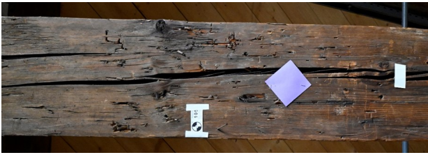
Figure 7. Examples of the real surface structure of historic timber with cracks, wooden knots and processing marks.
