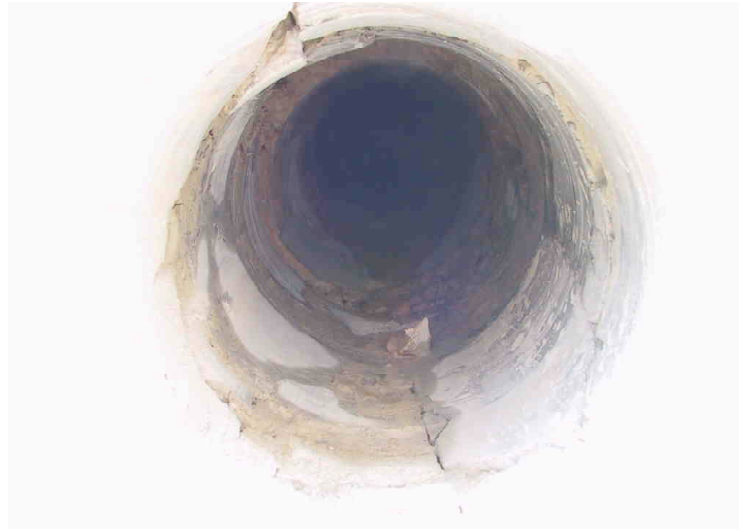
F 433 Blick in Bohrkernloch A 4 "Riss" 2003 S. Thole
