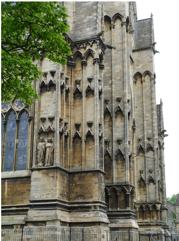
Ill. 17 Lincoln, Cathedral, Angel Choir, south-east corner with widely spaced bases and canopies on the buttresses
