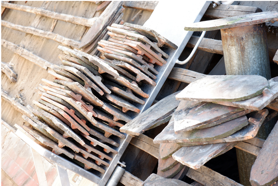
Figure 3. Salvaged tiles stacked on the roof of Georgenstraße 53b, Amberg, ready to be transported into storage (2023). Source: Courtesy of Jana Scherm.
