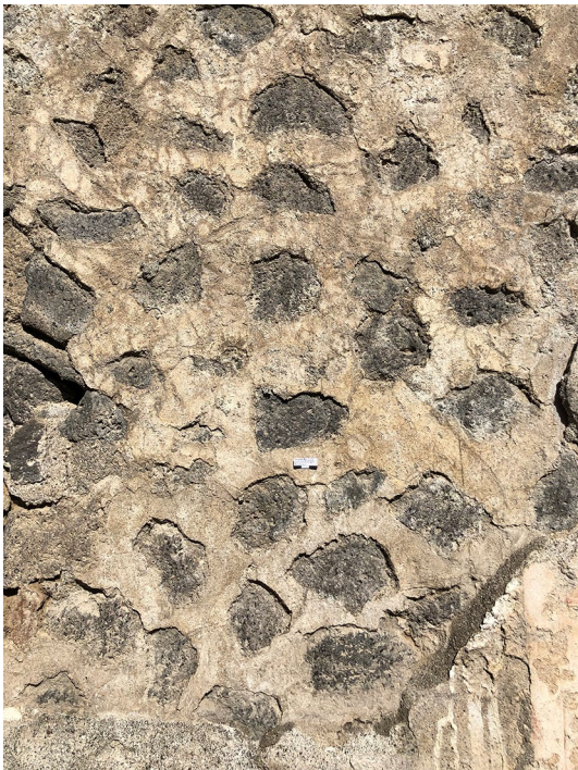
Fig. 5 Tomb PN-EN10, south facade. Detail of the lava stone cladding mostly covered by the lime jointing mortar
