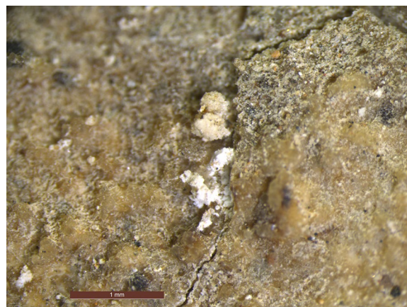
Fig. 21 Detail under microscope of the gypsum crust at the surface of a sample of a brick from the facade south of tomb PN-EN06. The surface is bulged and cracked. White salt crystals from subflorescence can be seen in the crack
