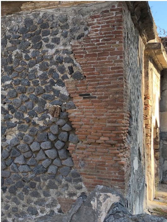
Fig. 4 Tomb PN-EN10, west facade. Detail of the corner chain made of terracotta tiles disposed according to the "a vela" technique
