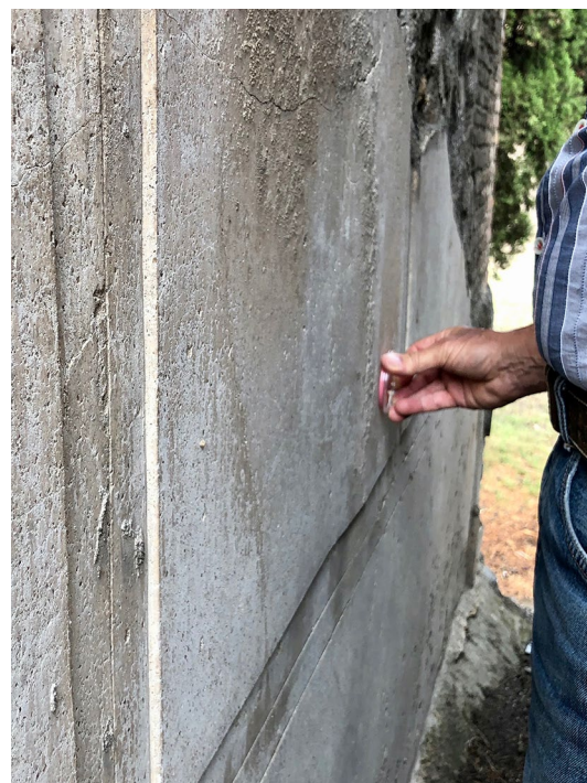
Fig. 10 Tomb PN-EN12, East facade. Measurements of Water Capillary Uptake using Contact Sponges in the intonaco render layer
