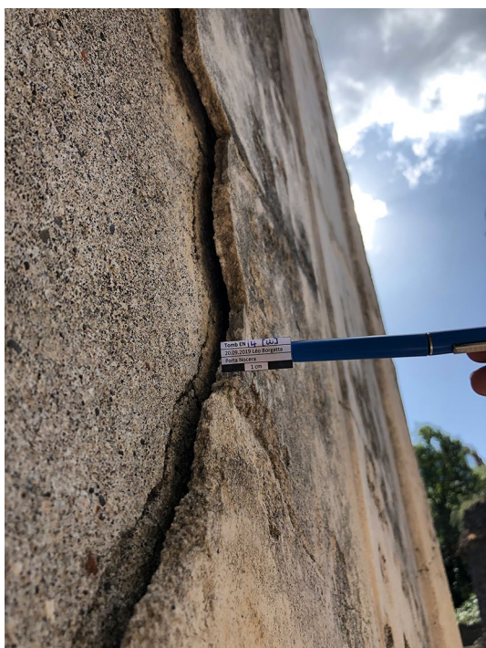
Fig. 26 Tomb PN-EN14, west facade. Detachment of the intonaco render layer from the arriccio with ca. 0.5 cm gap
